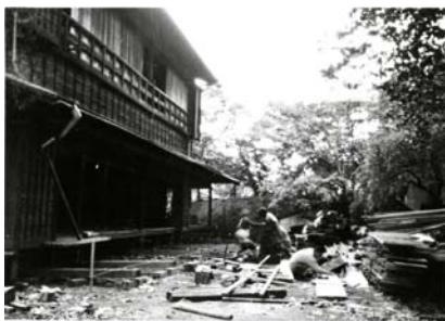
This picture from 1930 shows the dismantling of the former Akaboshi residence, prior to its relocation.
